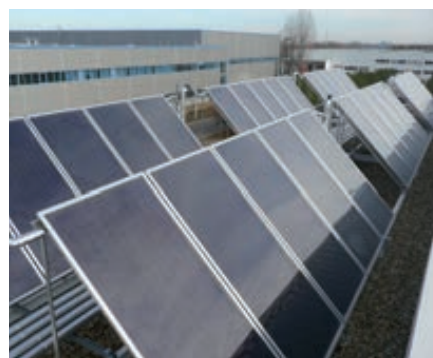
Hoval water heating system using solar energy.
